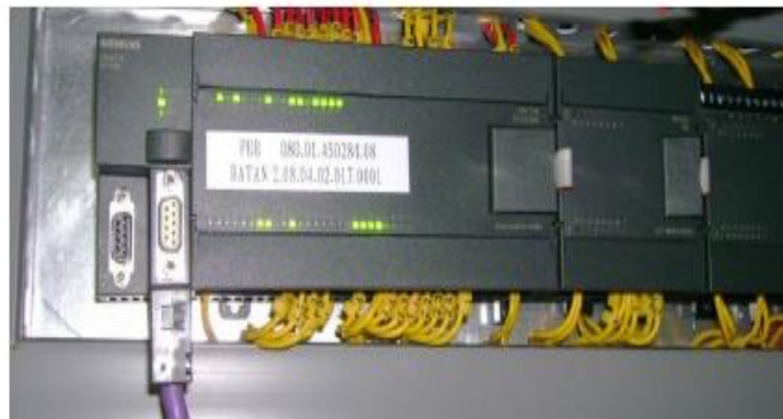
Fig. 3. Main controller of the safety system using the S7-200 PLC
