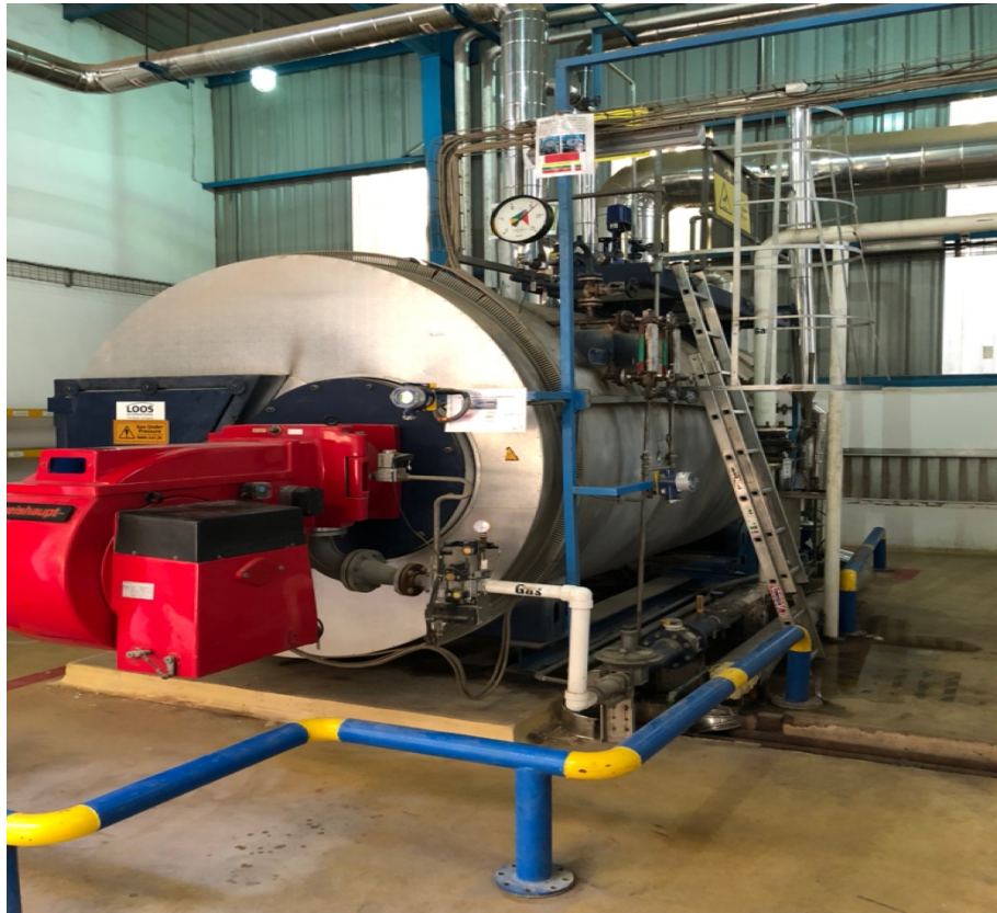
Fig. 2. Natural gas burner
