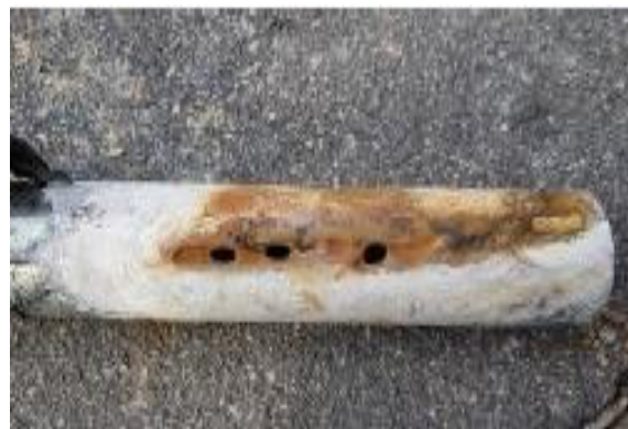
Fig. 1. Sample of corroded underground pipe
